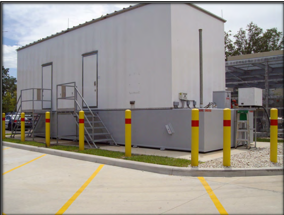
6. View of an emergency backup generator on the southeast side of the Sanford Fire Department/Police Department building at 1303 S. Lake Avenue.
