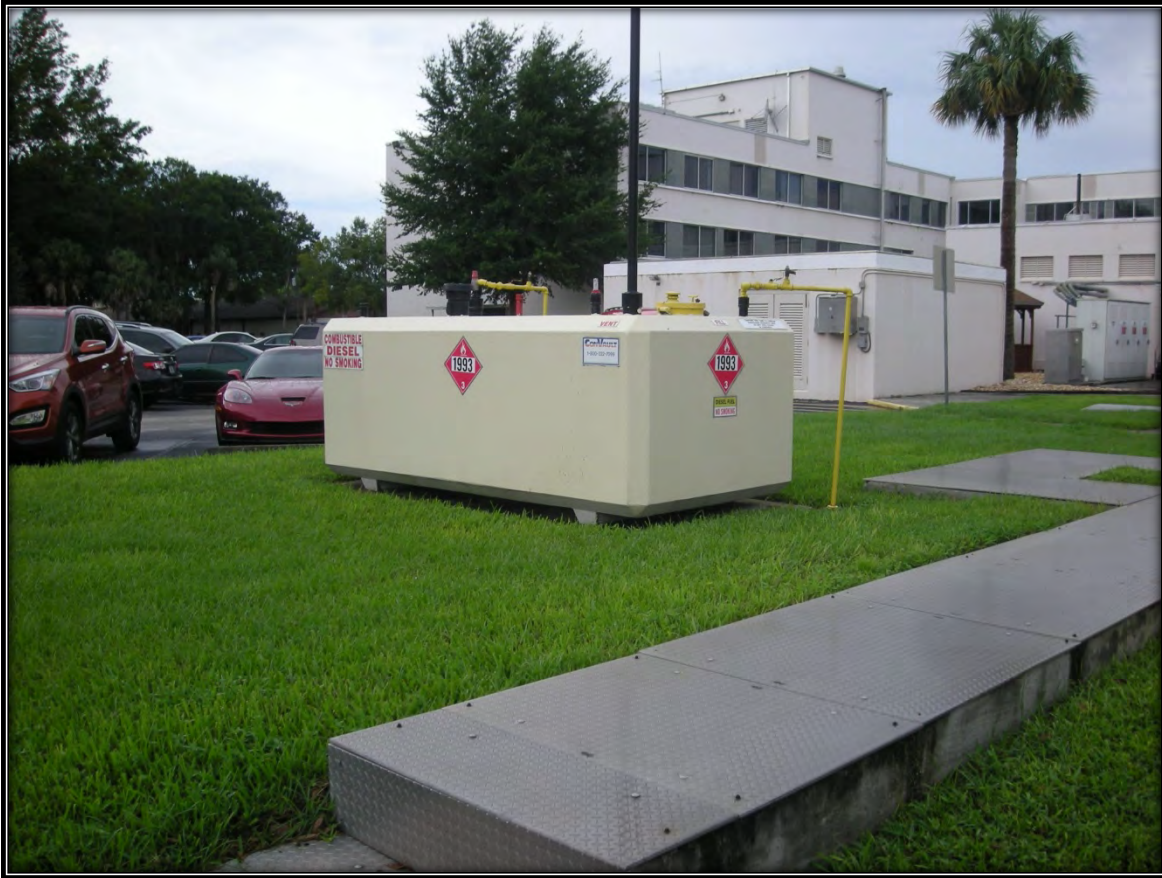
5. View of an approximately 2,000-gallon capacity diesel AST off-site to the north at 1101 E. 1 st Street.
